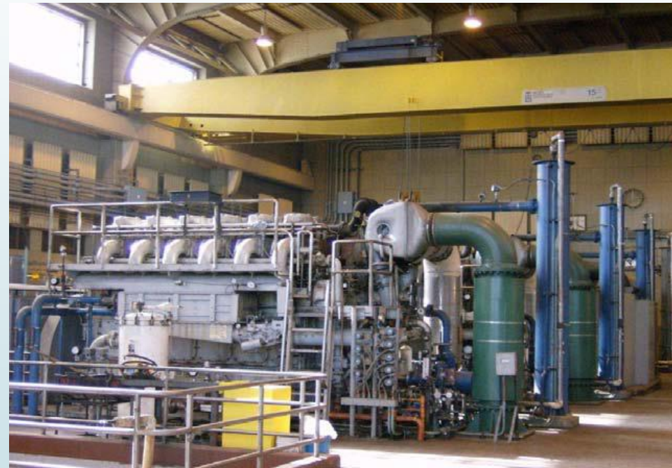
CHP system at Coney Island WRRF, NYC
