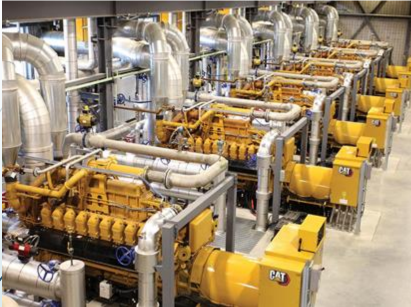
CHP system at landfill, Quebec
