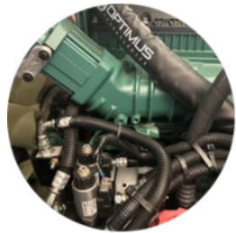
Fuel Selector Valves
